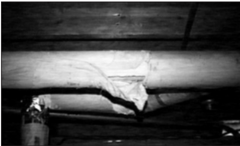
Minor Damage to Pipe Wrap
