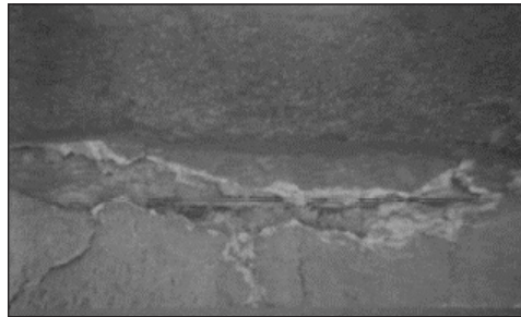
Major Damage to Fire Insulation
