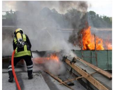
Fire caused by roofing operations
