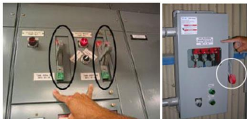
Disconnect panels with "lockout here" labels and energy isolation information
