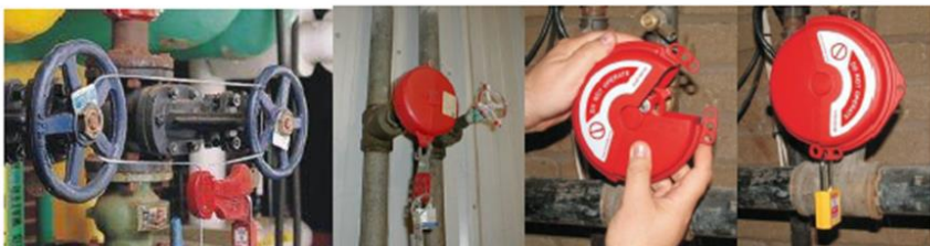
Piping shown "locked out"
