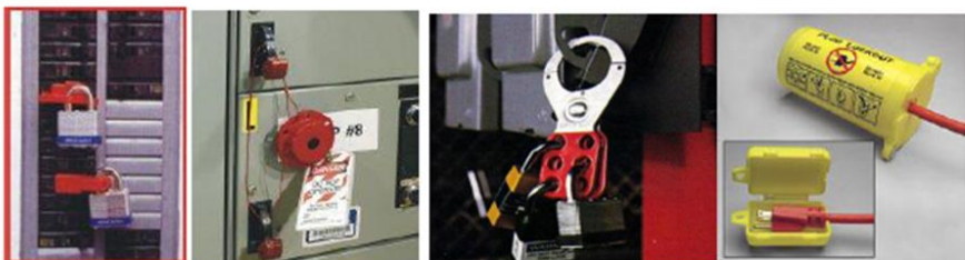
Electrical panels shown "locked out"
