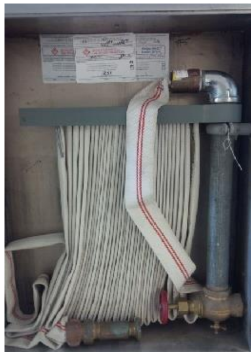
Charleswood School – Fire Hose Stand Pipe
